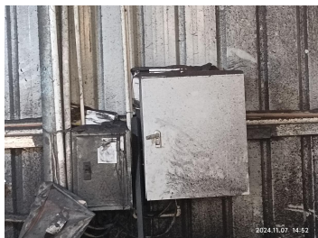
NC No warning sign.jpg
