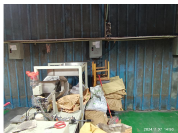
NC Blocked electricity box.jpg
