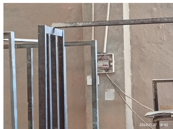
NC No insulation protective device.jpg
